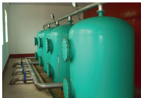
Water treatment facility in Liaozhong County, Liaoning Province
